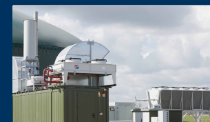
ElectraTherm Biogas Plant Trechwitz, Germany
